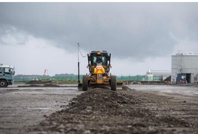
Groundworks at RNZAF Base Ōhakea as part of the infrastructure development to support the new P-8A fleet.
